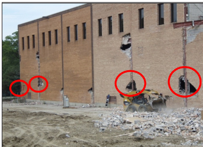
Figure 3. The Circled Columns on the North Side of the Building were Removed During the Experiment.
