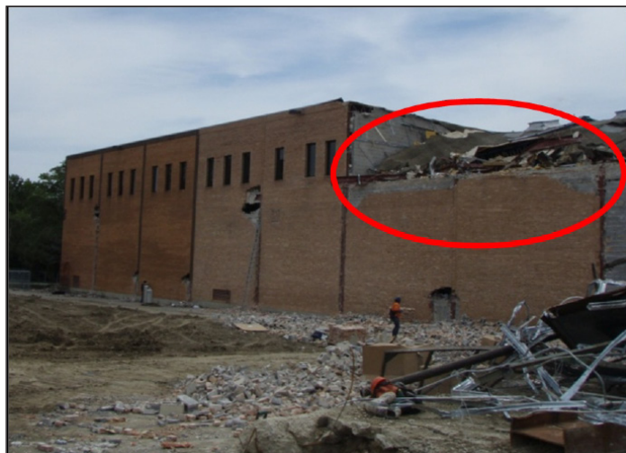
Figure 4. The Rubble Mass is Circled on the North Side of the Bankers Life and Casualty Company Building.
